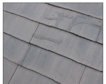
補修・塗装剥げ
